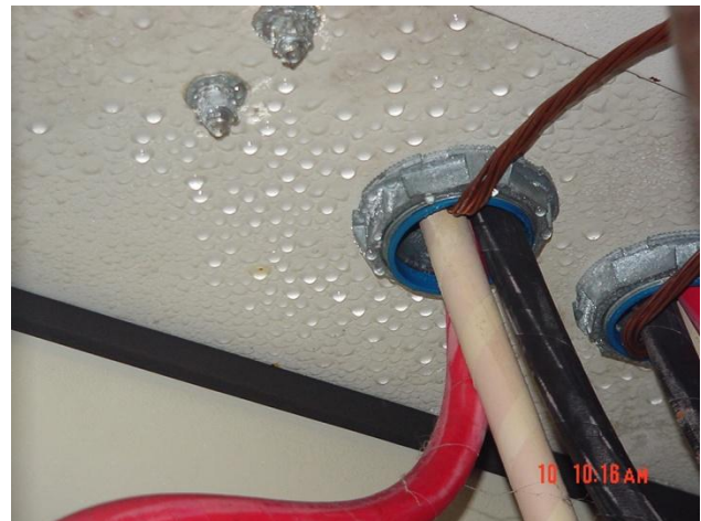
Figure 7. Condition that caused the unacceptable IRP
