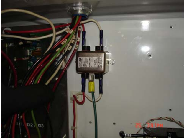
Figure13 – Line filters installed on a new controller.
