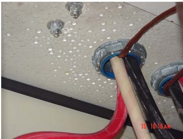
Figure 7 – Condition that caused the unacceptable PIP.
