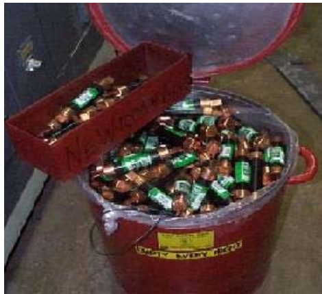
Figure 5- Failed 100 amp fuse graveyard for grinder motors.
